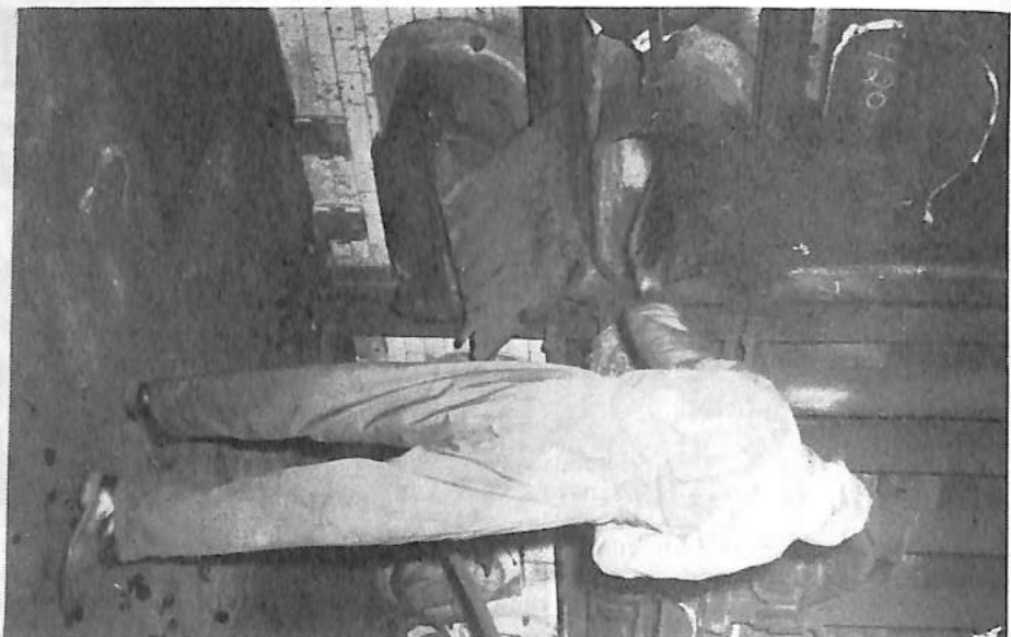
Charging a horizontal retort in Muirkirk Gas Works, August 1977
